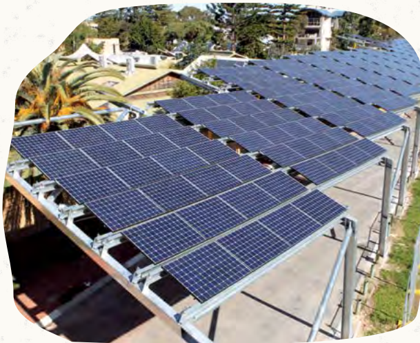
The solar array generated 290,000kWh of electricity.
